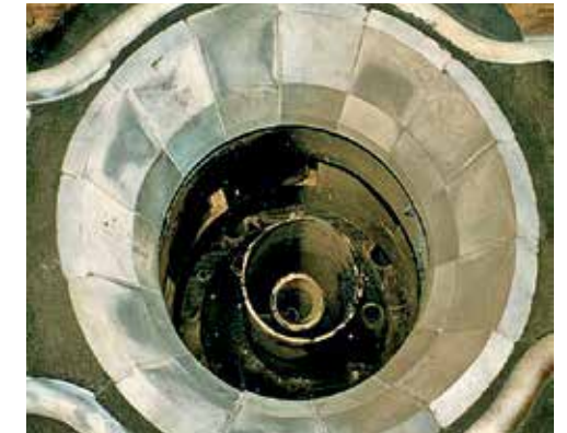
PF-burners reflectors protected by KALSICA N (photo) or KALMETALL.
