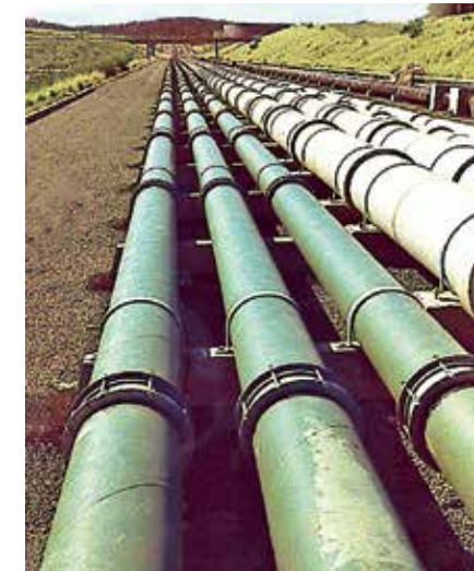
Wear protection for hydraulic and pneumatic pipes
