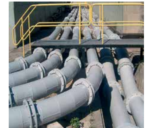
Pipes for several units running to the central disposal site in Brazil.
