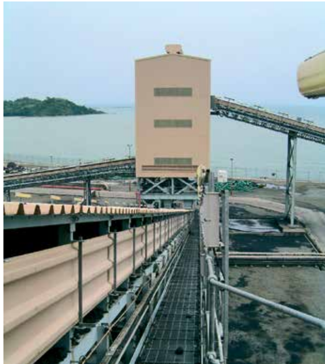
Coal transfer equipment is protected with ABRESIST fused cast basalt or KALOCER high alumina ceramics (example: Philippines).
