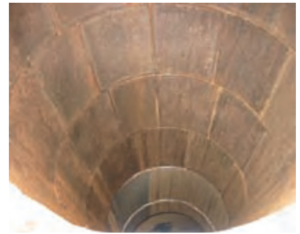
The abrasion-resistant basalt tiles in a cyclone's barrel section are larger than the tiles in the cone section.
