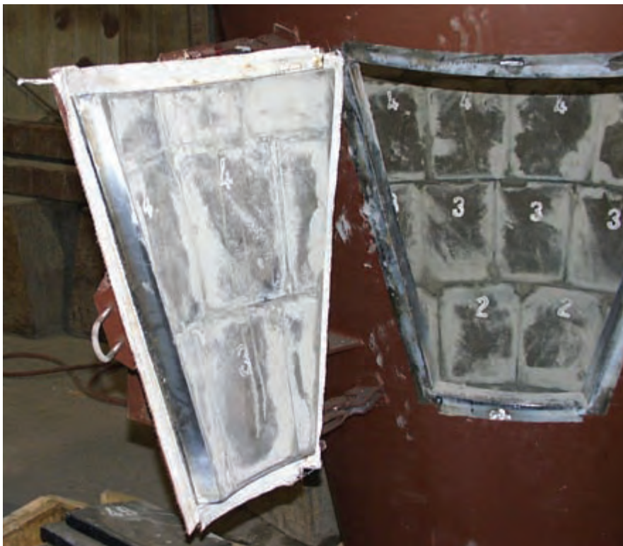
Abrasion-resistant basalt tiles line a cyclone's cone section.
