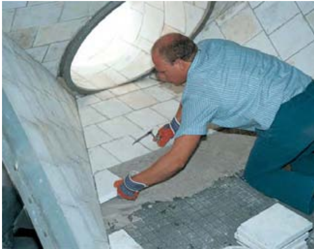
Collecting hopper being part of sintered material dust collection at 400° C/752 °F: effectively protected with KALCOR zirconium corundum
