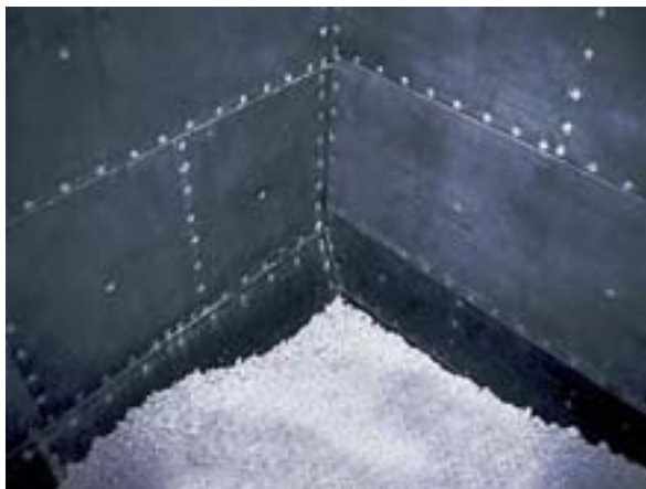
Raw meal bunker with slide promoting lining made of KALEN-1006
