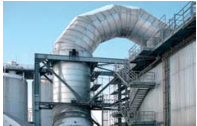
Clinker dust pipe protected with KALCRET hard compound
