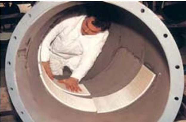
Dust collecting pipe for clinker fitted with 6 mm thick KALOCER mosaics set in KALFIX epoxy adhesive
