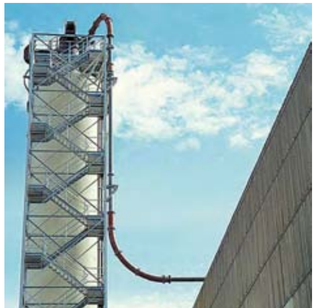
Transport pipe to the cement silos; the bends are protected by ABRESIST just like the straight extensions
