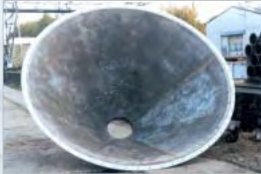
Lining the separator of a ball mill used by the cement industry with KALCRET-BNX hard compound
