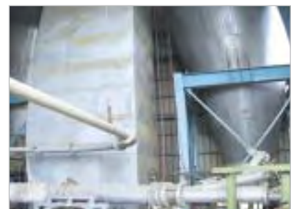
Lined cyclone in a cement plant
