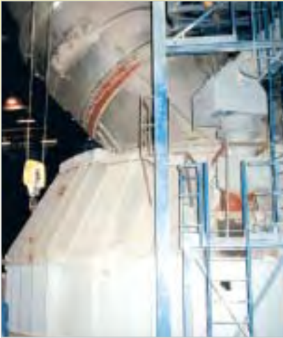
Lining of a raw meal grinding mill in a cement plant
