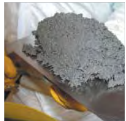
6. The stiff/plastic KALCRET compound (X) to be applied by trowelling is compacted with the aid of a vibration trowel
