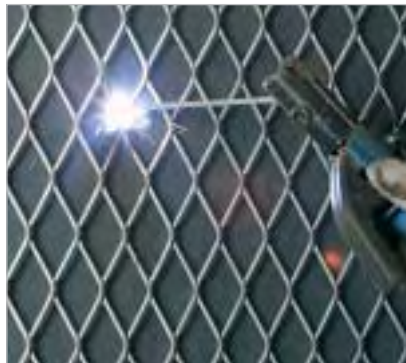
Welding the wire mesh to the surface to be lined: distance approximately 250 mm
