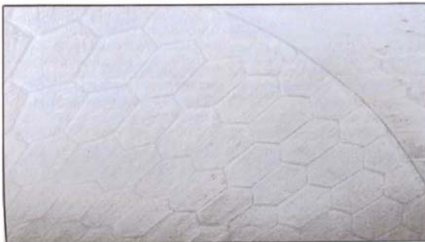
A close-up of the basaltic lining inside the air separator shows very little wear after three years, as evidenced by the fact that the honeycomb pattern is still quite visible. Each tile is 1 ¼ in. thick.
